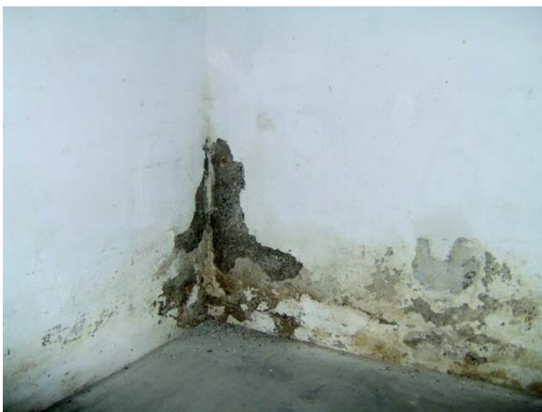
Dampness in Kiseljak Ammunition Depot building, which currently stores ammunition. Officers in charge pointed out that they needed materials to bring the buildings up to safety standards.
